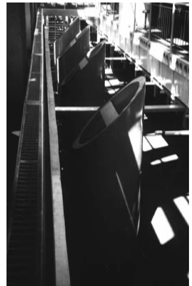
Floor mounted return silencers.
