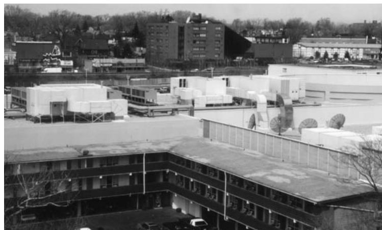
Hotels surround rooftop units.
